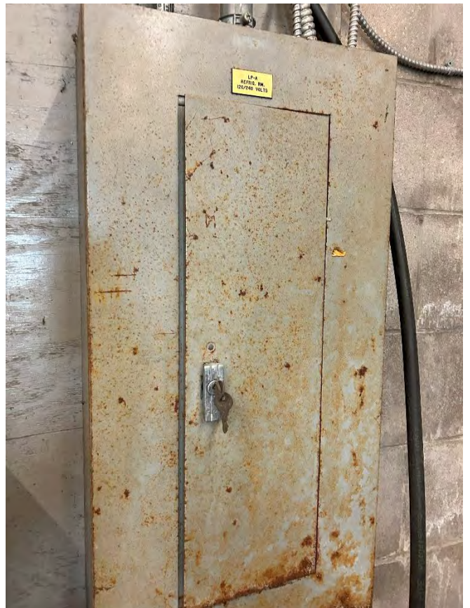
Sample Electrical Panel to be replaced
