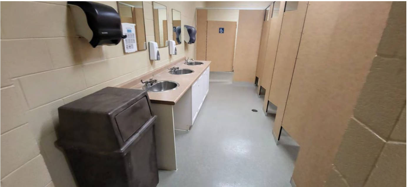
Community Center Washroom Fixtures
