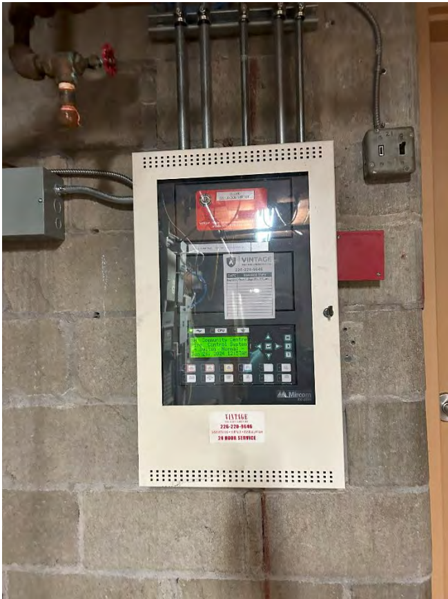
Existing Fire Alarm Panel
