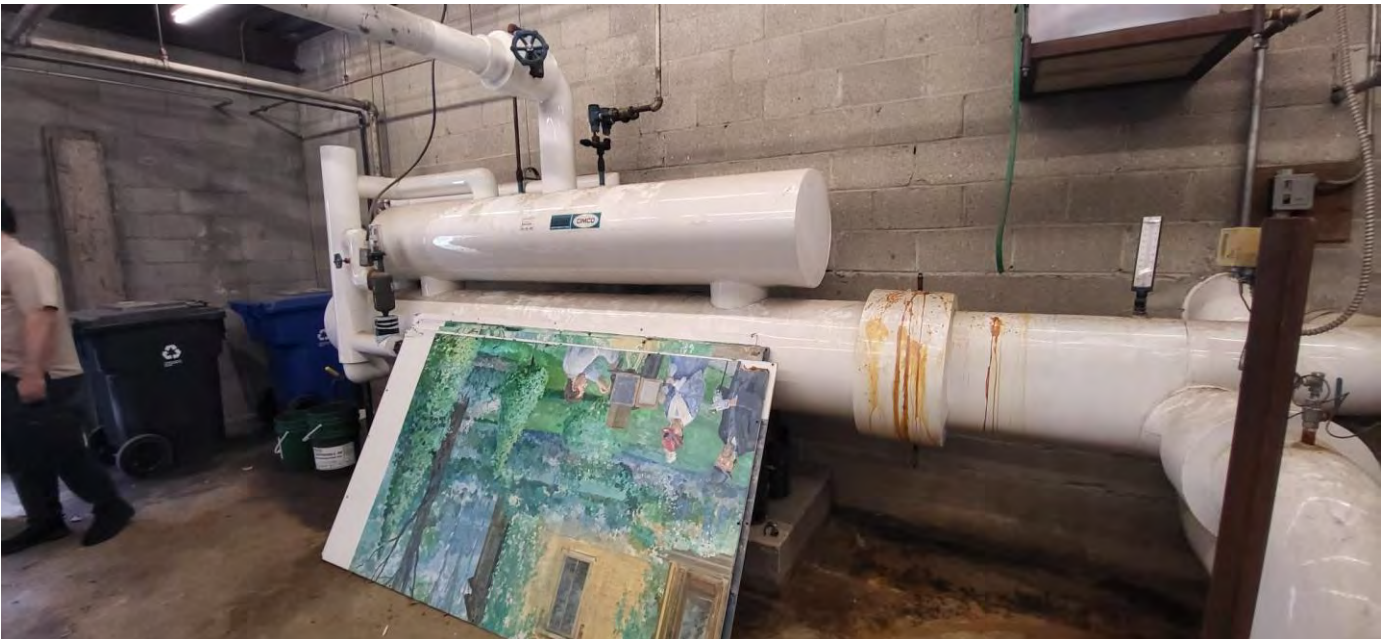
Ice Plant Shell & Tube Chiller
