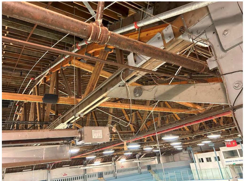
Wiring Run Exposed
