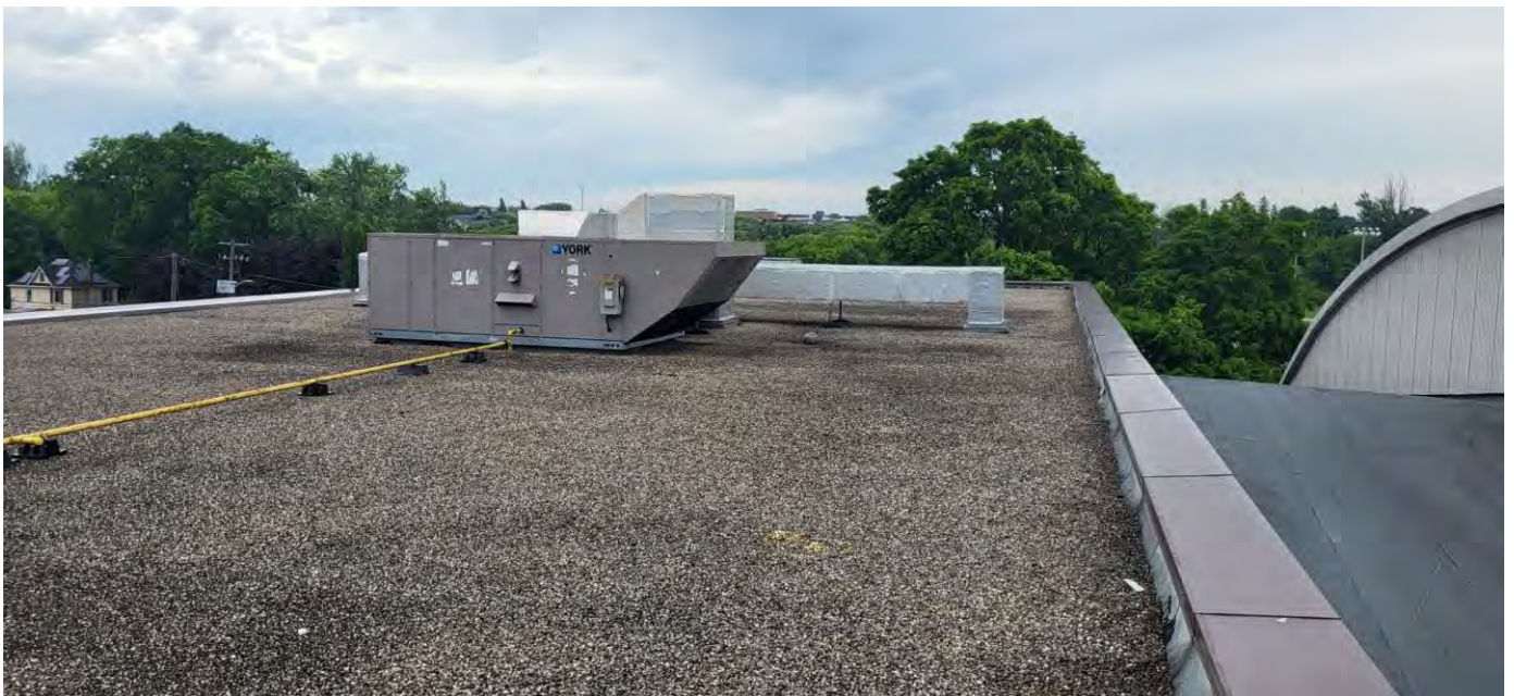
Community Centre Multipurpose Room HVAC Unit
