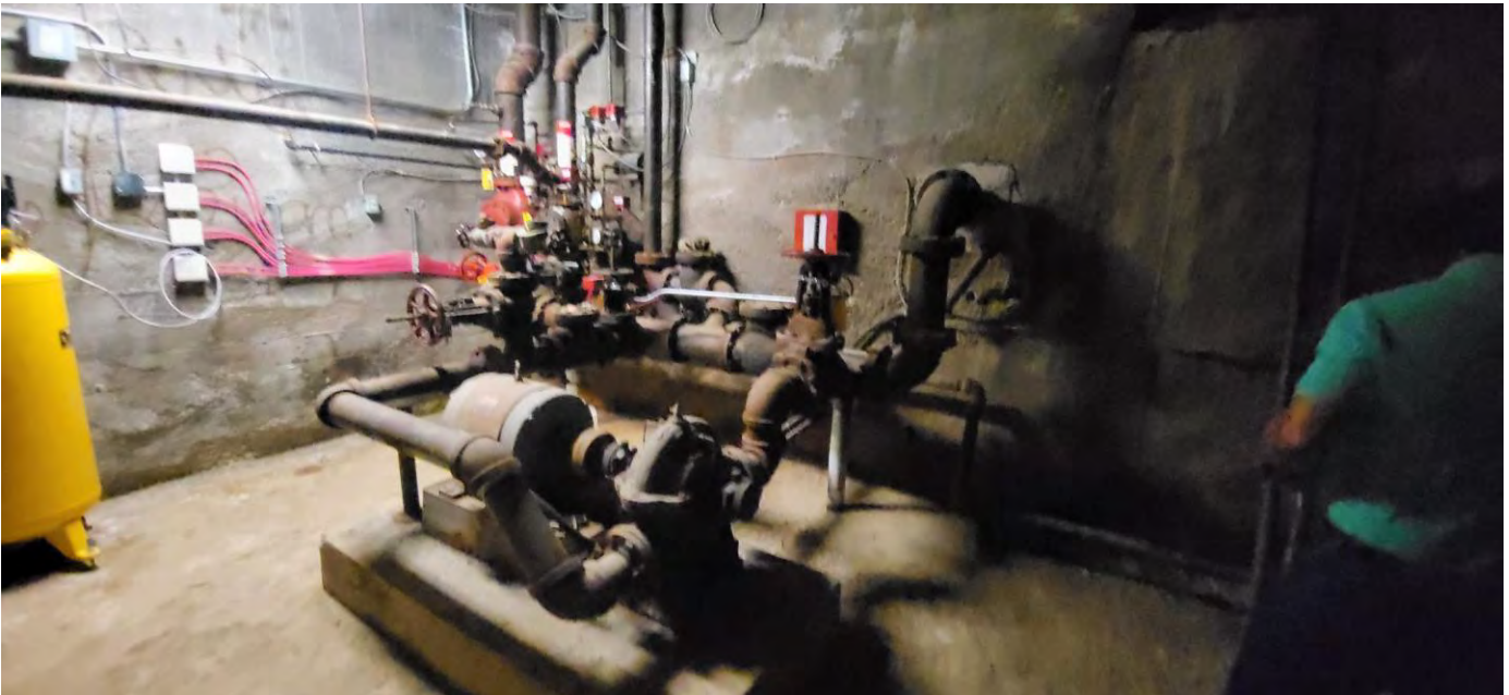
Fire Pump and Wet Sprinkler Header
