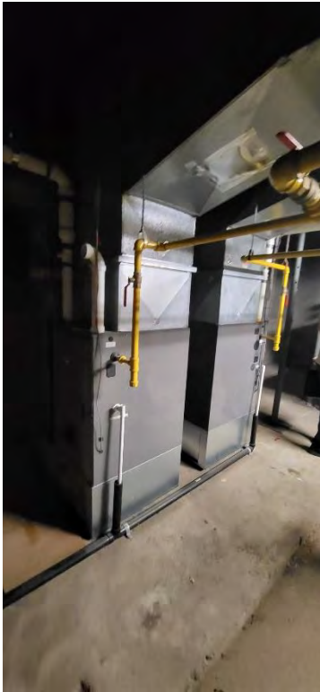
Gas Fired Heating Furnaces
