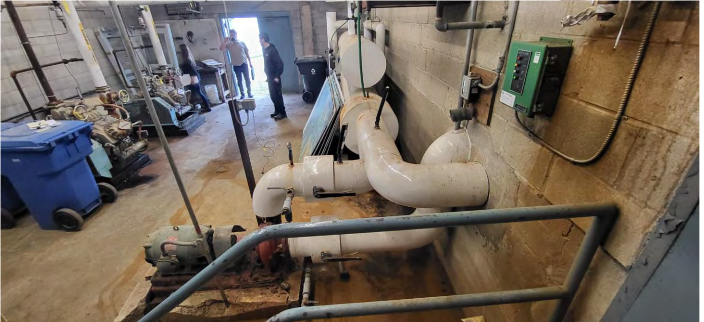
Refrigeration Room with Brine Pump
