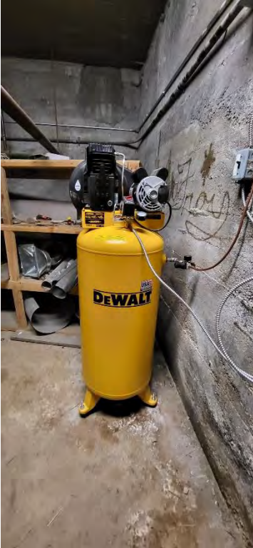
Dry Sprinkler Air Compressor
